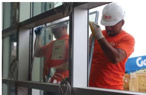
Installers from Pal's Glass Service Inc., www.palsglass.com , set electronically tintable glass and make the electrical connection for the glass at the Siemens' wind turbine facility in Hutchinson, Kan.
