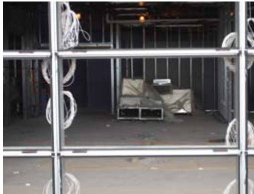
Fig. 5. The openings are prepared and ready to accept the electronically tintable IGU. The setting blocks are in place, the frame wire harnesses have been pre-run and holes are sealed.
